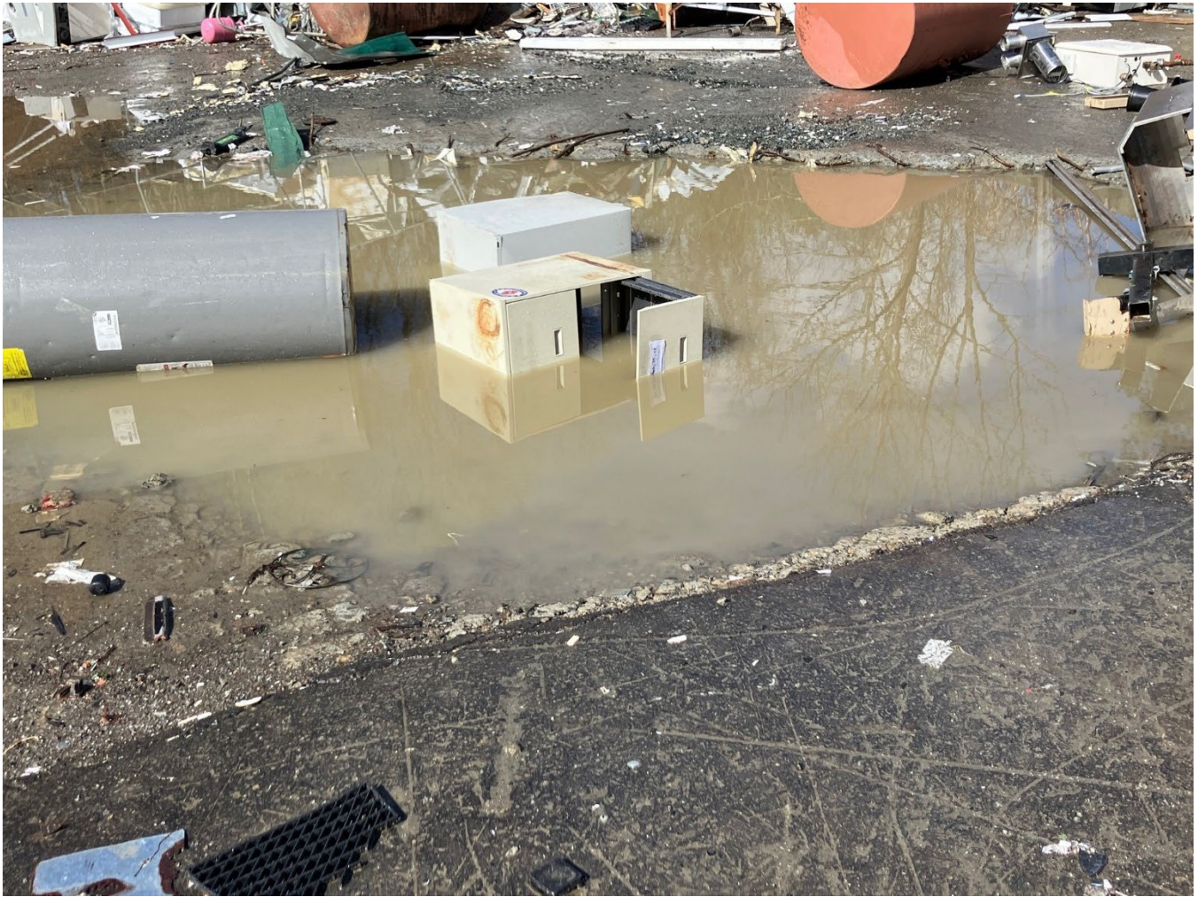
ABOVE: One of two areas in the current scrap metal pad that has degraded enough to hold water. Exposed rebar is also visible along the top of the 'lake'.
